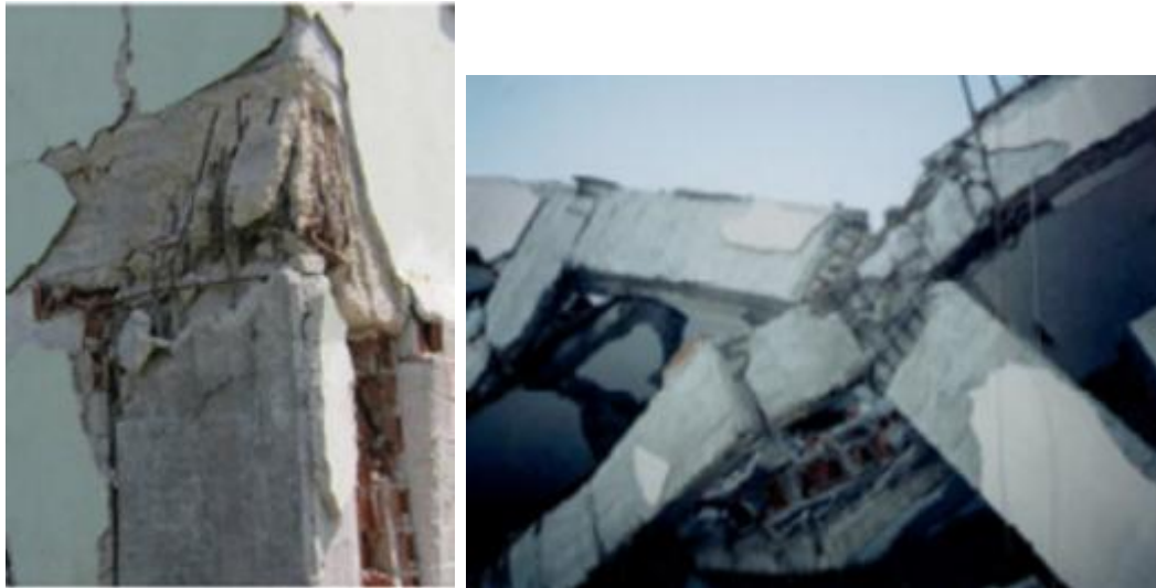
Imagen 5. Daño en unión viga columna fuente: construction and design defects in the residential buildings and observed earthquake damage types in turkey.
