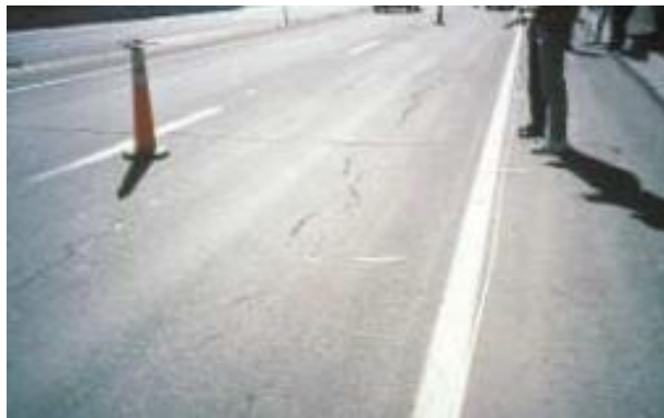
Figura 9 Piel de Cocodrilo. Deterioro Leve, Fuente Distress Identification Manual for the Long-Term Pavement Performance Program
