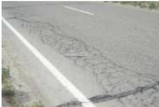
Figura 11 Piel de Cocodrilo. Deterioro Severo, Fuente Distress Identification Manual for the Long-Term Pavement Performance Program
