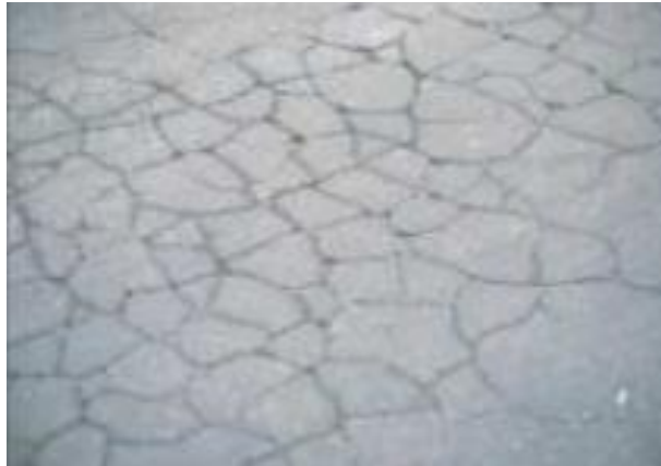
Figura 8 Piel de Cocodrilo. Fuente Distress Identification Manual for the Long-Term Pavement Performance Program
